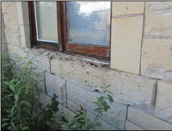
Rotted windowsill on west facade
