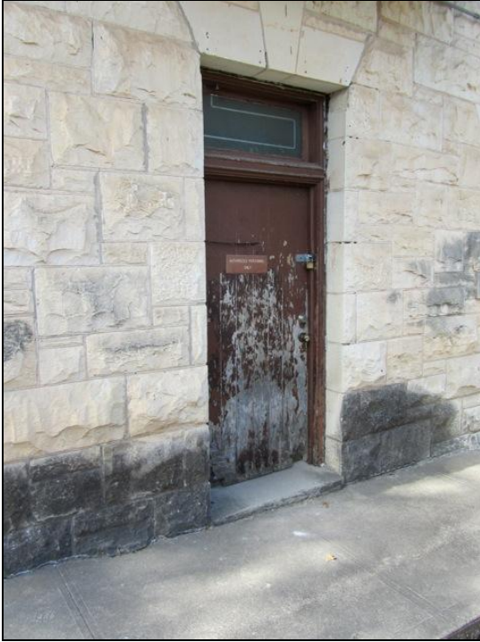
Rotted wood door on north façade
