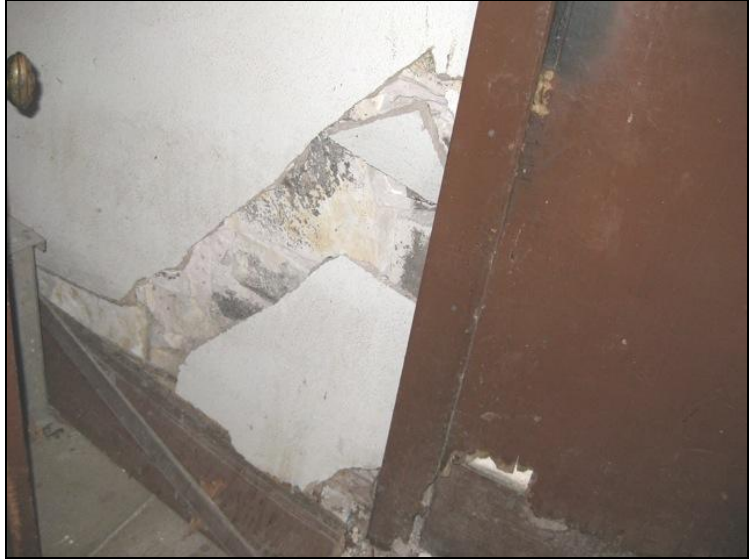
More plaster damage
