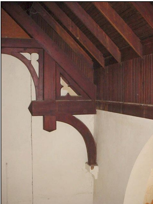
Water stains on interior wood
