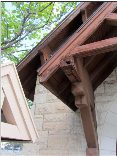
Rotted wood bracket
