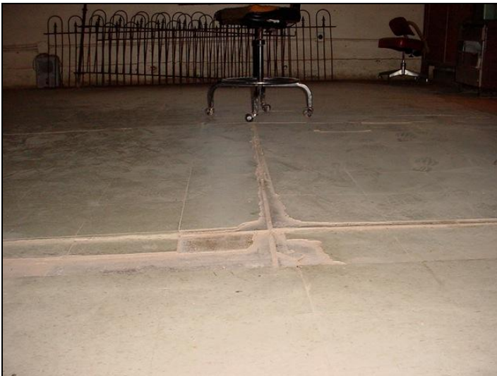
Uneven floor surface with asbestos tile (SAC Photo)
