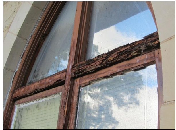
Rotted frame and sash on east facade
