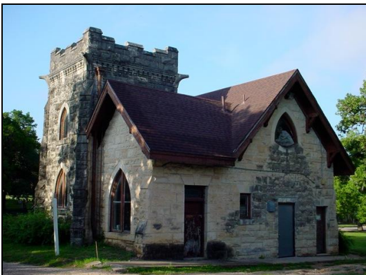
Mildew stains on tower and north wall of chapel
