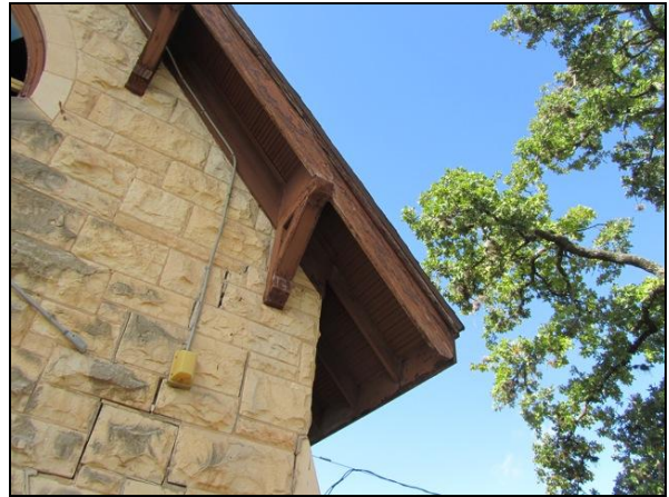
Surface mounted electrical
