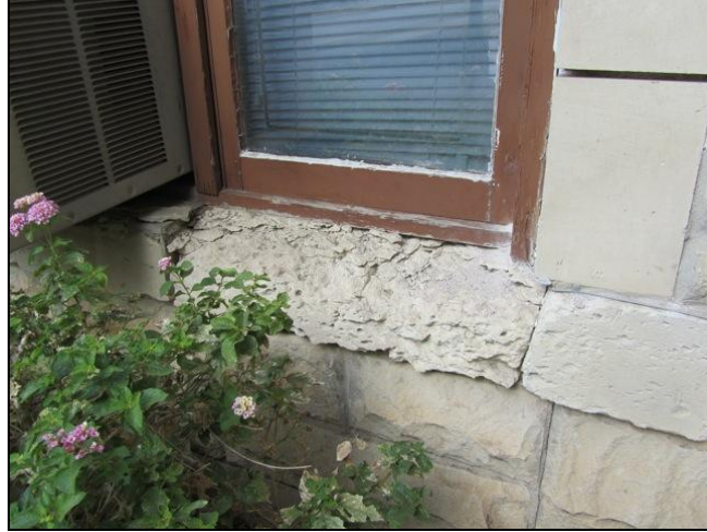
Open joints and badly deteriorated stone sill
