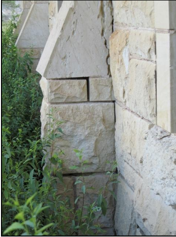
Open joints & displaced stones
